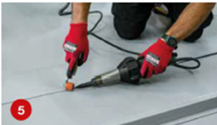
5. Hot-weld the 180mm wide membrane cover-strap to seal over the fixing line, taking pressure off the existing membrane.
